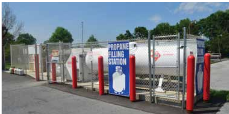
The Propane Filling Station is a great add on for attended washes.
