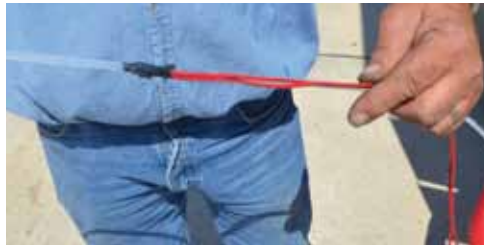
Step 12: Now it is time to feed the power lines and the air tube up through the channel. By taping these lines together, it makes it easier to thread.
