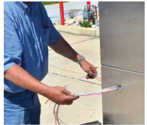
Step 10: Thread the new wires, pick up lines and air hose through the the hole.
